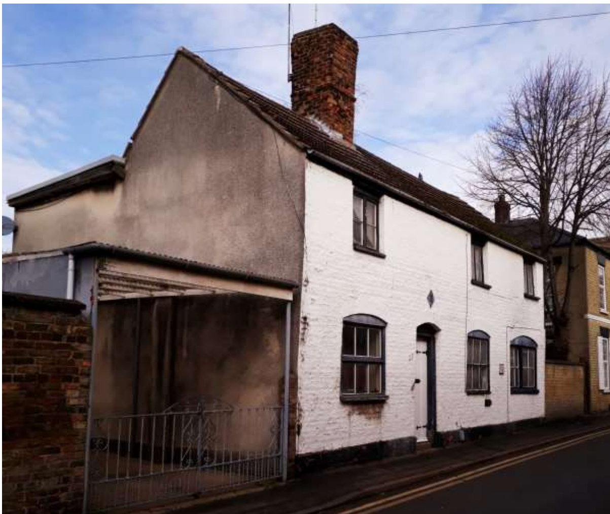
20-22 St Mary's Street is probably the oldest surviving building on the street but its front elevation and stack are in need of repair and maintenance.
